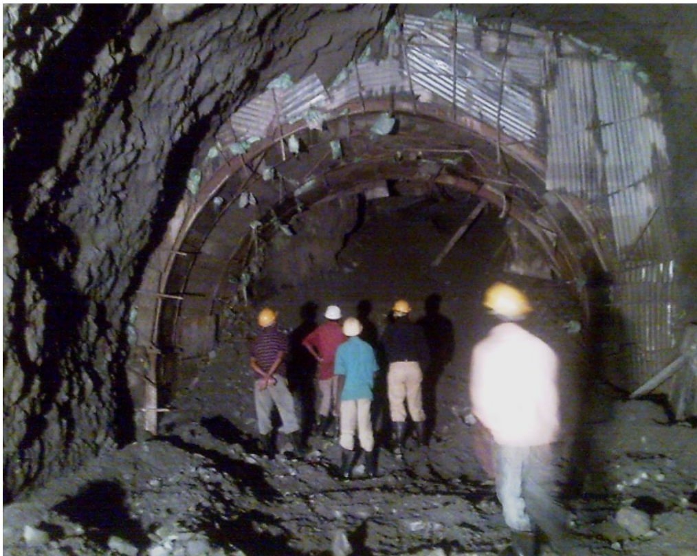
Figure 2 Loose muck flowing from the 15 m high chimney at RD-1940 m
