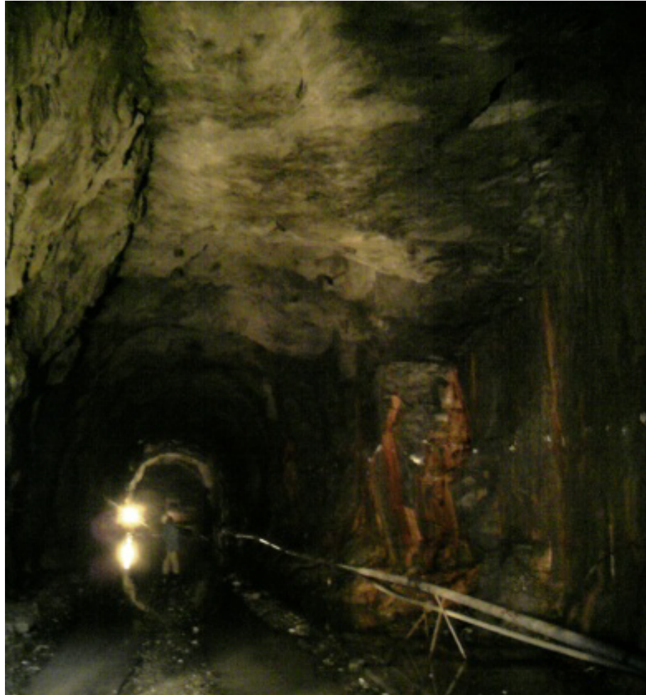
Figure 3 Over breaking along shallow dipping joint in the crown portion and Sub-vertical cross joint on the right wall
